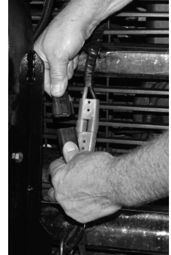
All electrical connections cleaned and add dielectric grease once/month
